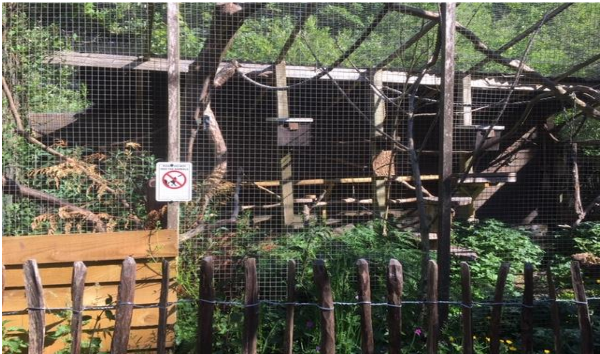
Plate 12 - Hoarding container along the back of the old side of the Breeding Enclosure
